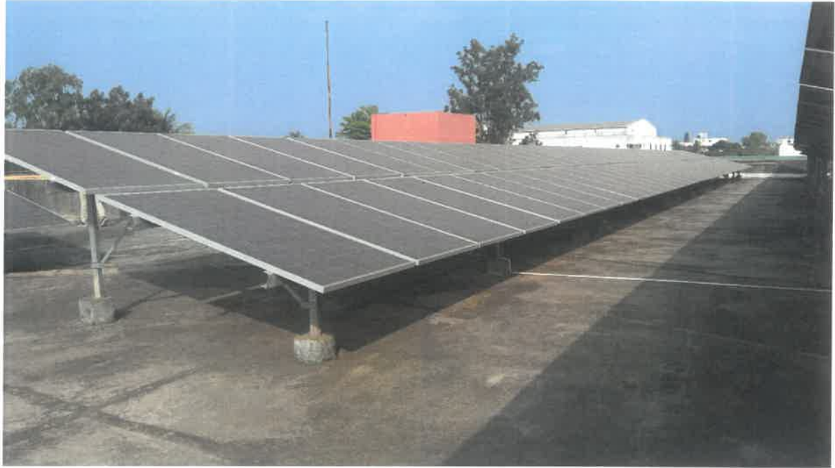
Solar panel on roof of Laboratory building
